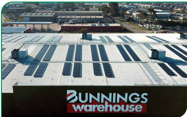
Bunnings' hundredth on-site solar PV system
