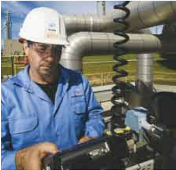
Mechanical Fitter Kevin Gohrt monitors vibration at the export pumps.
