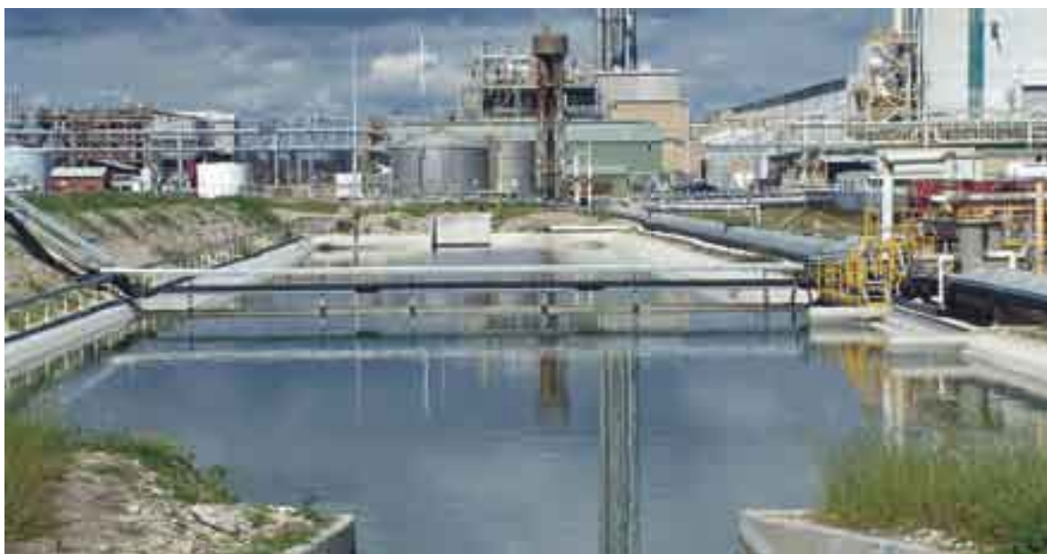
Effluent recycling ponds at the Kwinana site store liquid waste until it can be reused in the fertiliser manufacturing plant.
