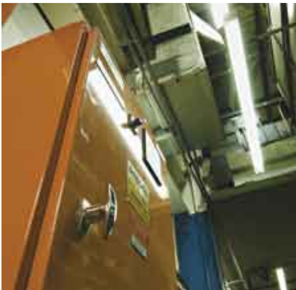
Power factor unit at Bakers Construction and Industrial, Blacktown, New South Wales.
