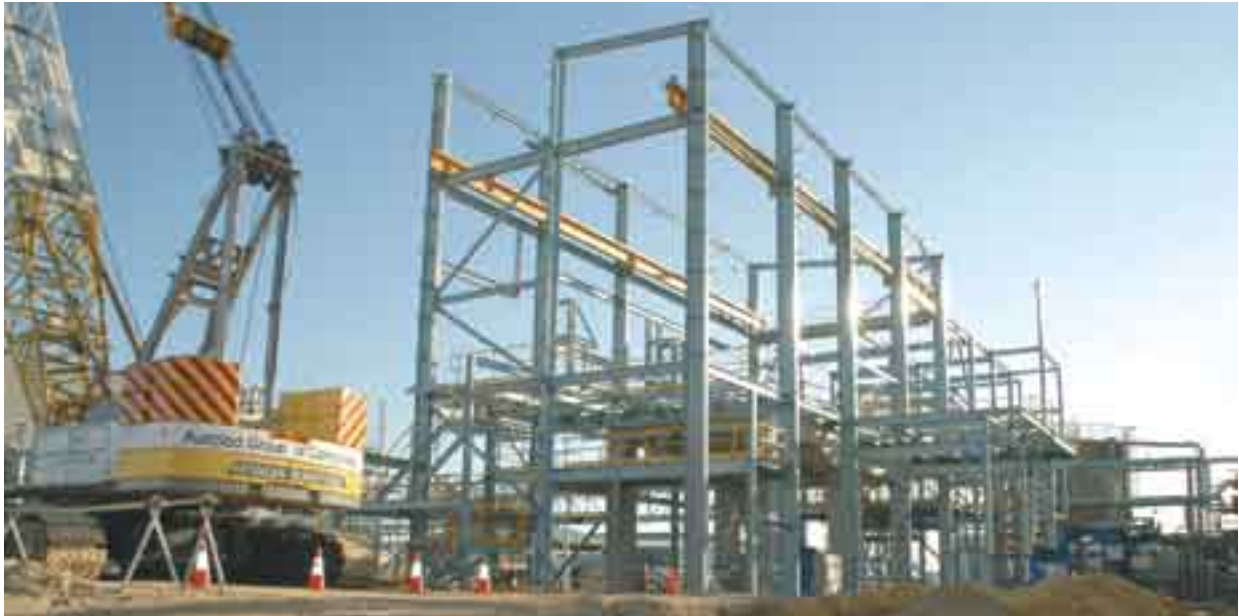
Structural steel work for the new nitric acid and ammonium nitrate plants.
