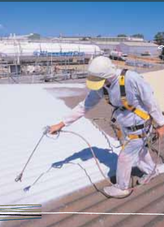
Spraying fibro seal to encapsulate asbestos roof sheeting at the LPG terminal, Kwinana, Western Australia.
