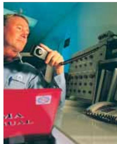
Operations Supervisor Garry Tardrew testing the Kwinana Industries Mutual Aid (KIMA) radio in the plant's central control room.
